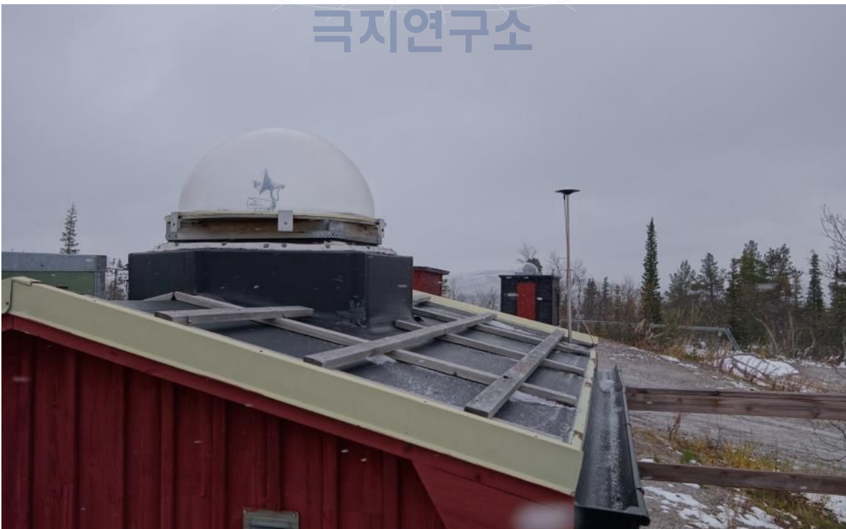
Fig. 56 GPS receiver installed at ESC, Sweden
