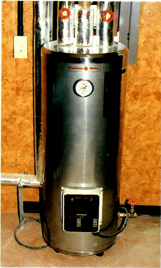
Fig. 8. Hot water supply heater for each building.
